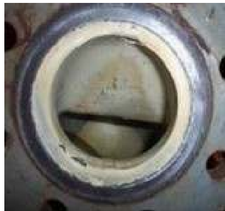
Pipe Interior After Treatment
